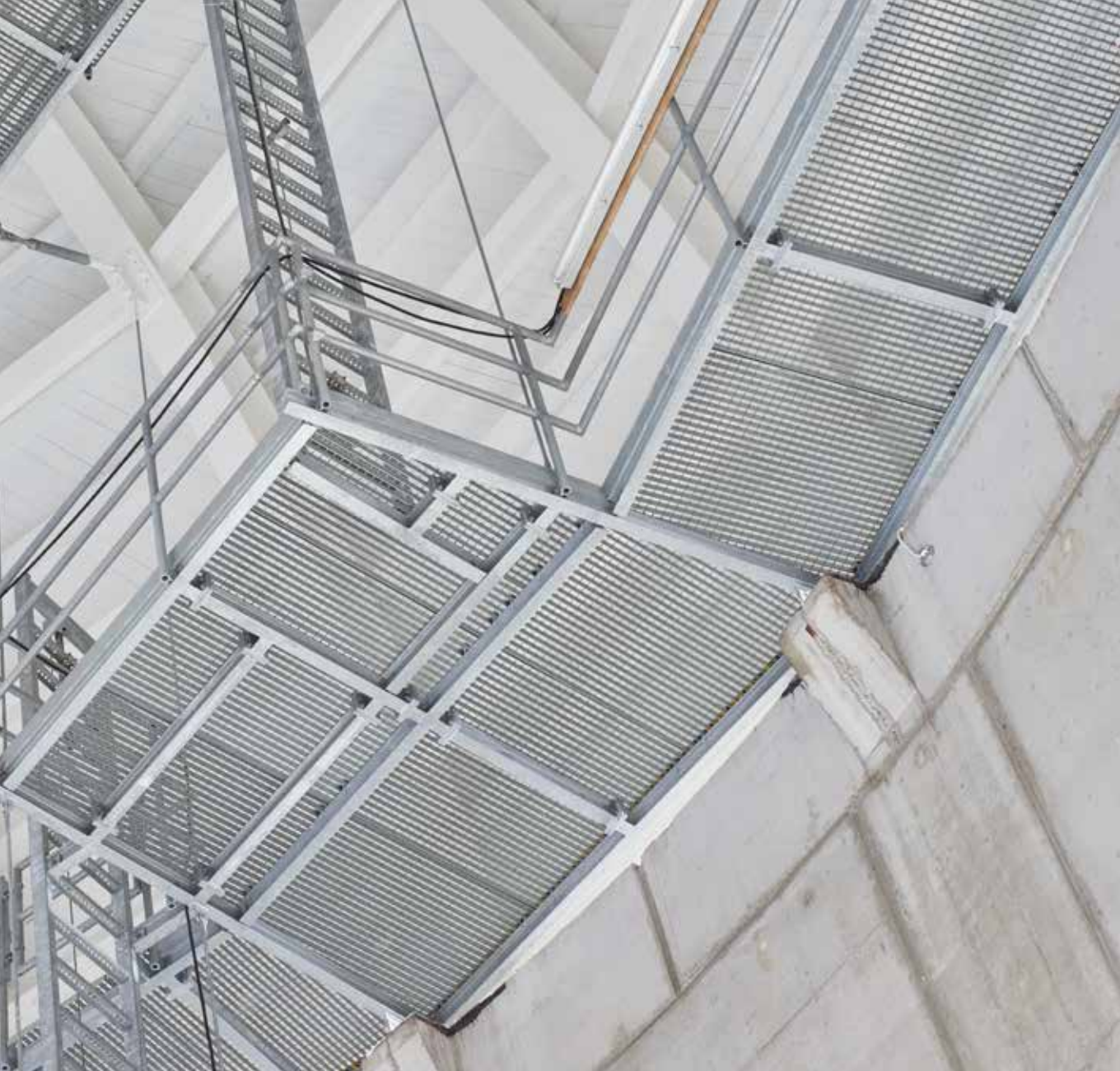
CELLULOSIC ETHANOL PLANT, STRAUBING
